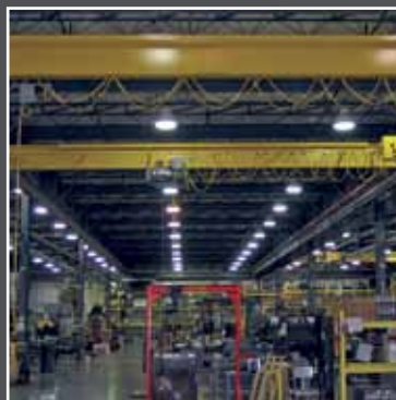
Festoon System on an EOT Crane, USA
