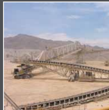
Festoon System on a Traveling Hopper, Peru
