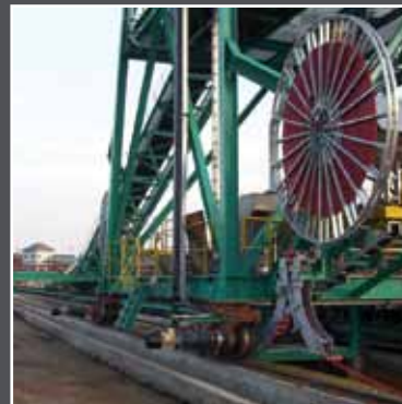
Motor Driven Cable Reel on a Stack/Reclaimer, Thailand
