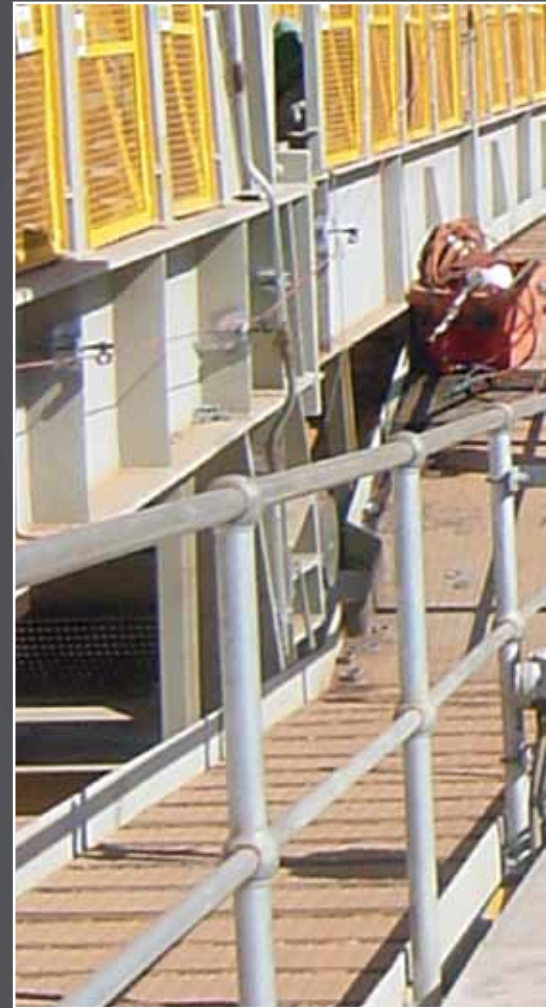
Level Wind Reels on a Stacker/Reclaimer, Australia
