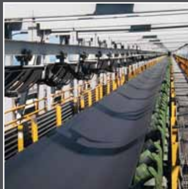
Festoon System on a Tripper Conveyor, Venezuela
