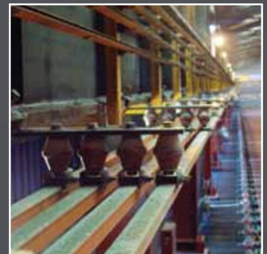
"Dura Coat" Conductor Bar System on an Electrowinning Process Crane, Chile
