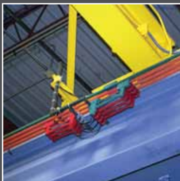
Conductor Bars on an EOT Crane, USA
