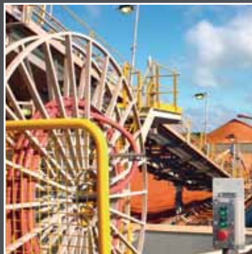
Motor Driven Cable Reel on a Stack, Australia
