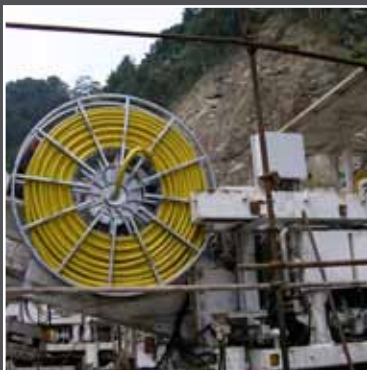
Motorized Cable Reel on a Tunnel Boring Machine, India
