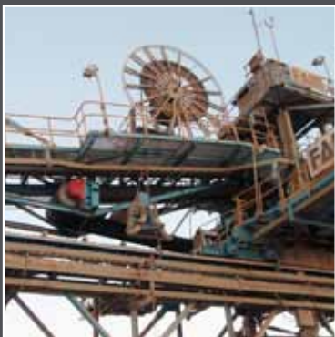
Motor Driven Cable Reel on a Tripper, Chile
