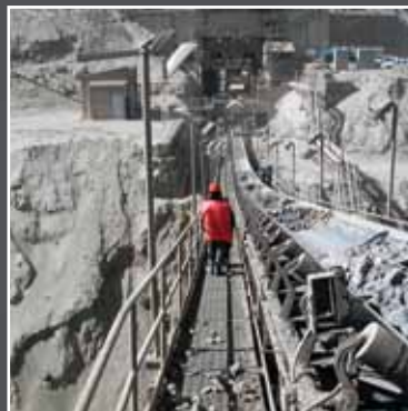
Festoon System on a Conveyor, Chile
